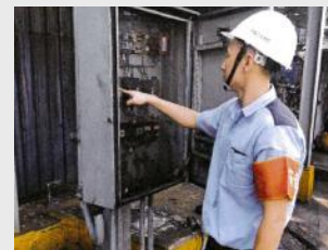
Safety protection class: Initiate the plant safety protection facilities
