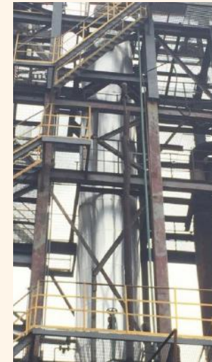
Overall heat exchange section
