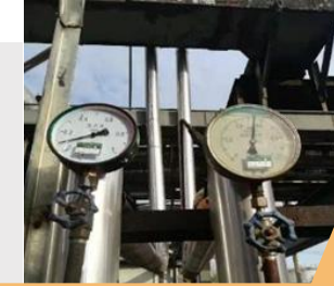
Pressure gauge without verification label was improved
