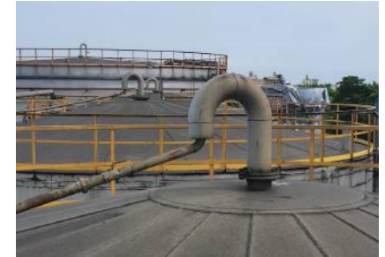
Breather valve connecting pipe setup
